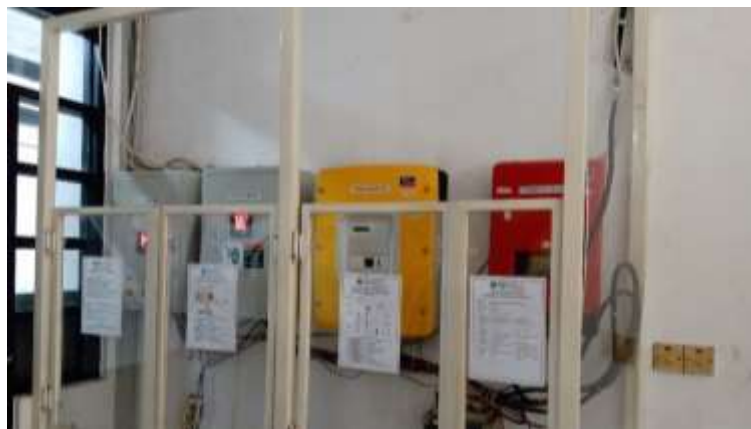
Implementasi Baterai Energy Storage System di Smart Microgrid Labtek VI - TF – FTI
