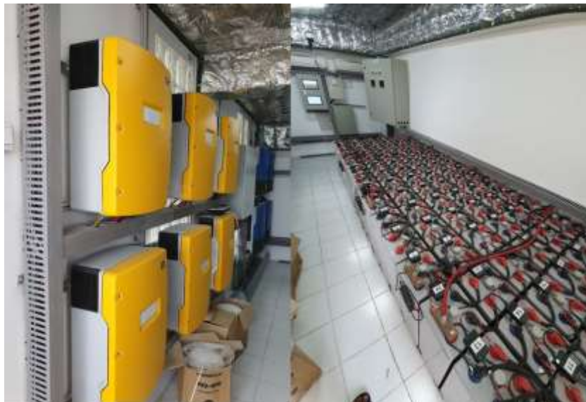
battery energy storage system di smart microgrid Gedung Labtek XIV SBM-ITB
